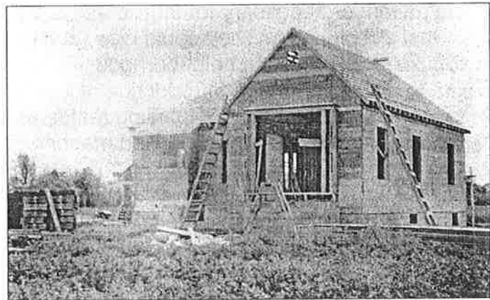
Single-family residence under construction in the Sunny Lea housing development. Photo courtesy of Lane County Historical Museum (GN2026)
